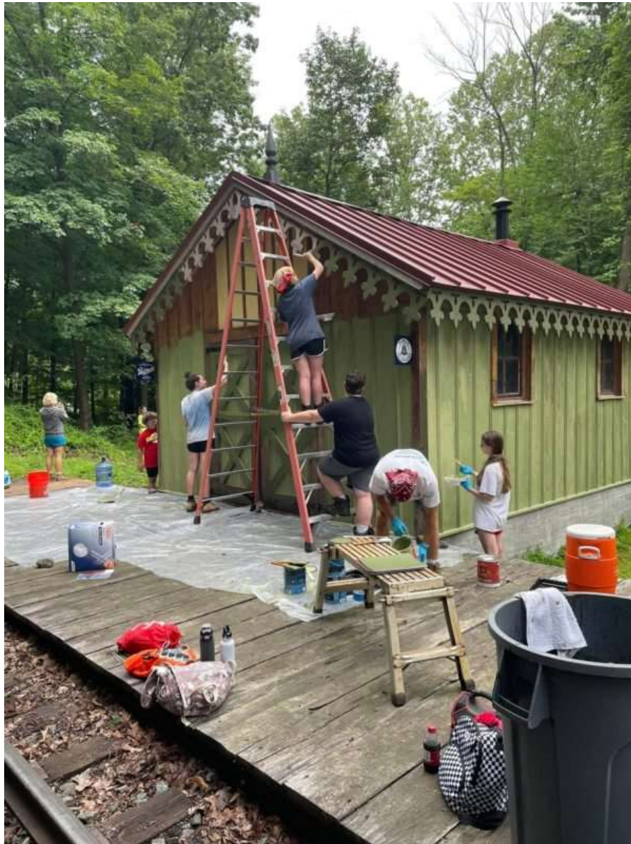
Volunteers work on building structures at the old Colebrookdale ironmaking village site, which will also be home to the Colebrookdale Children's Educational Grove.
